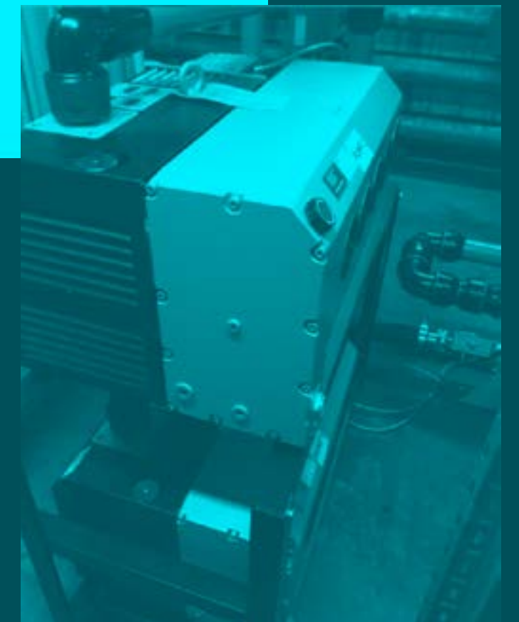
Implementation of compressed air dryer vacuum pumps
